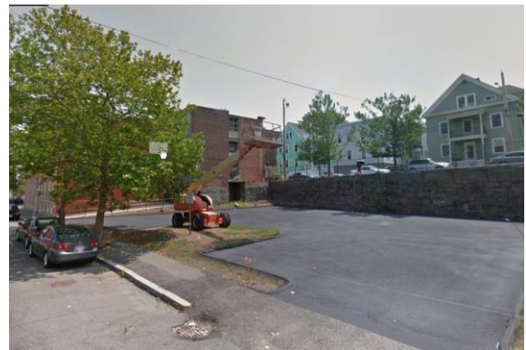
34 Peabody Street is slated to become Lighthouse 34 with the construction of 21 affordable housing units.
