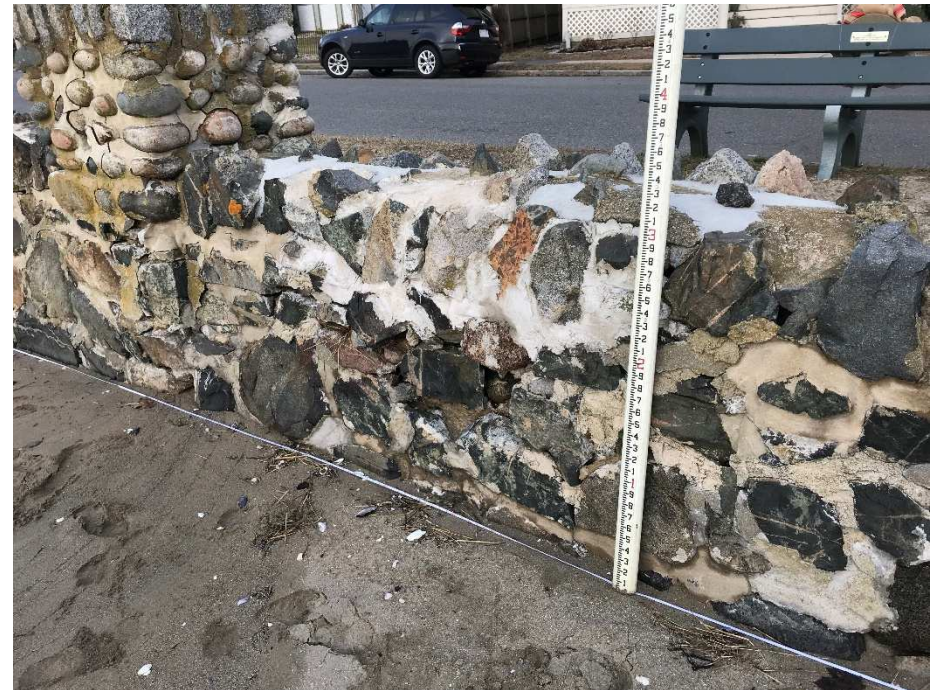
Missing face stones and typical recent mortar repair.
