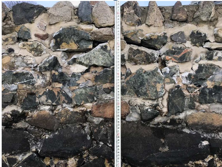
Typical voids and missing mortar along seaward face.
